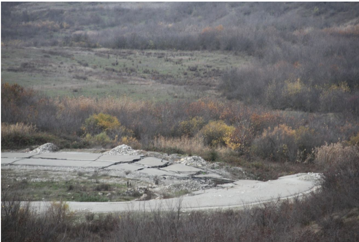
Figure 1: Road Destroyed by Landslip (Mughanli-Ismayilli. 2012)
