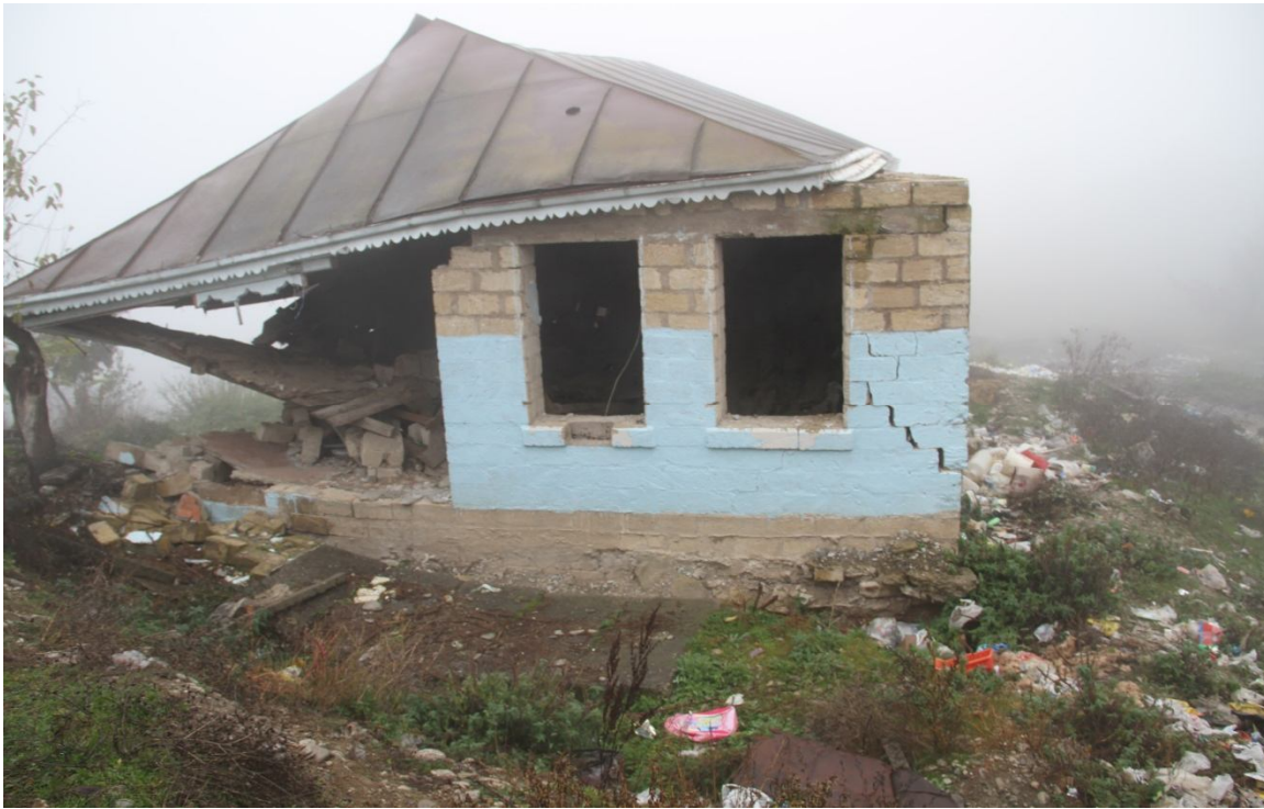
Figure 2: The Home Destroyed by Landslip in Mughanli Village
